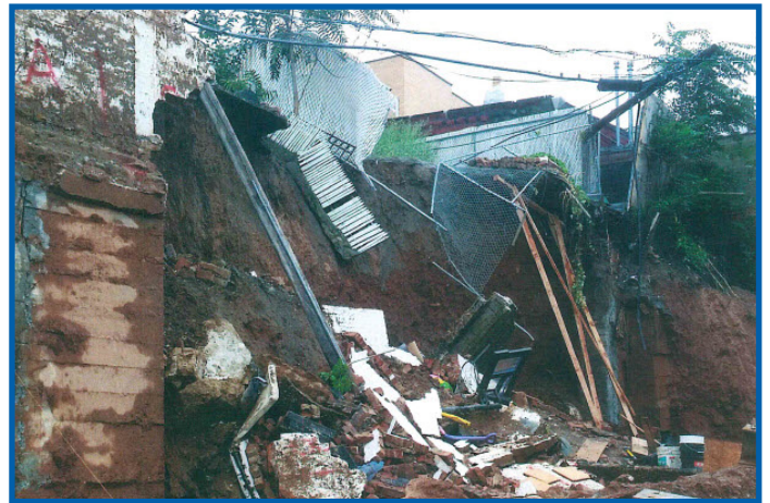
Aftermath of wall collapse
